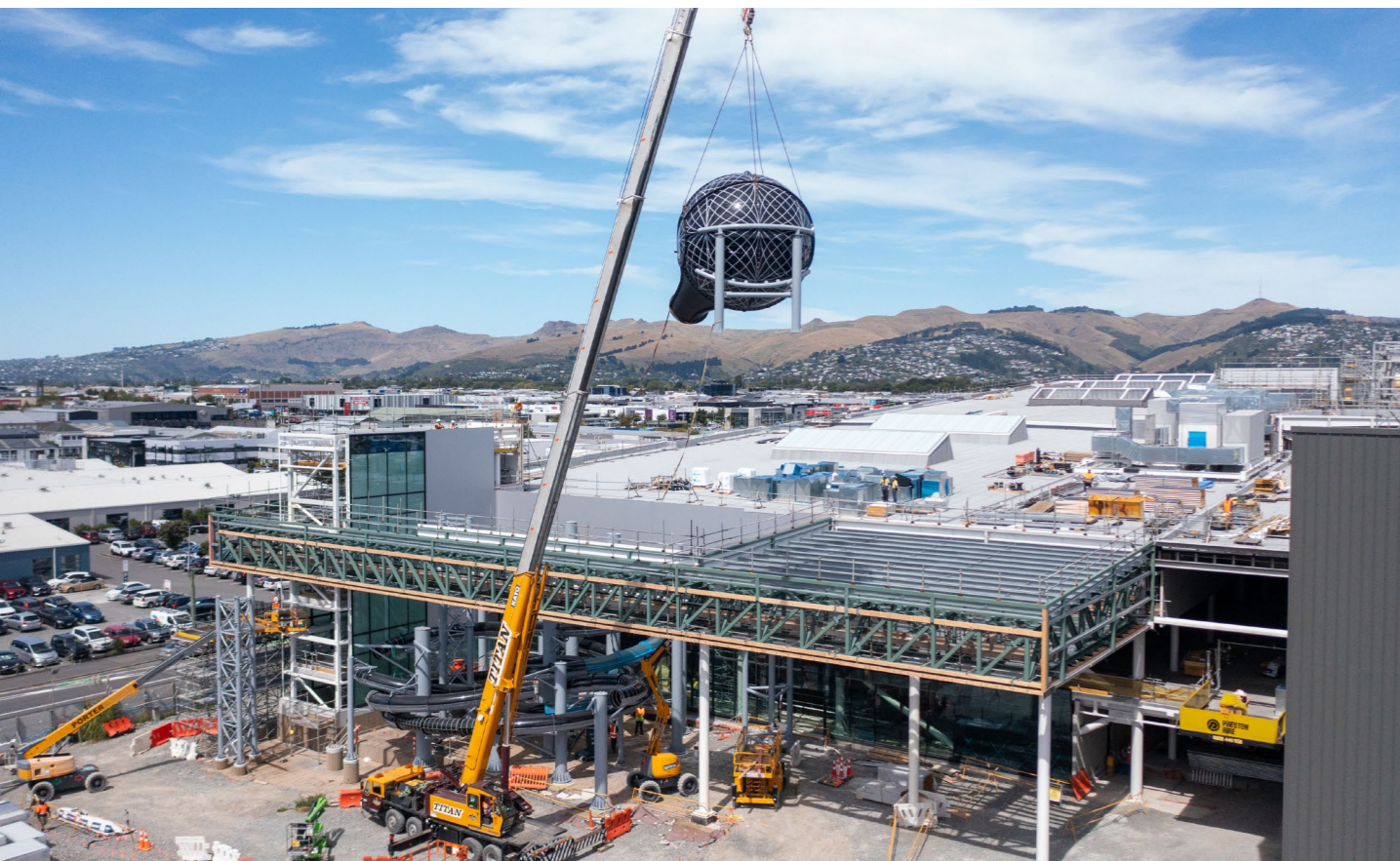
The large sphere for one of the hydroslides was lowered into place at Parakiore Recreation and Sport Centre.
